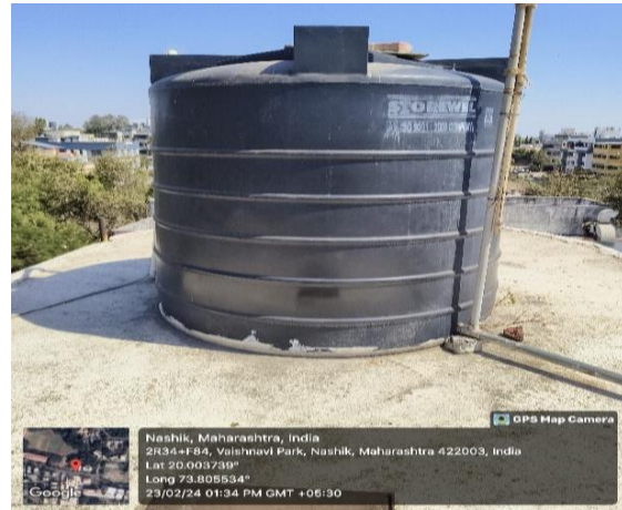
Overhead Water Tank – Boy’s Hostel
